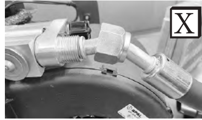
Improperly Seated O-ring Land
