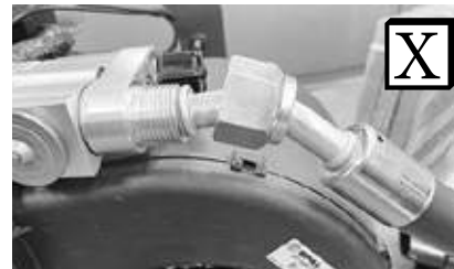
Improperly Seated O-ring Land
