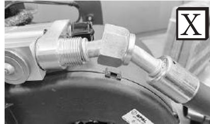
Improperly Seated O-ring Land
