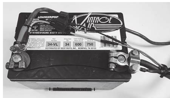
Completed Installation Shown
